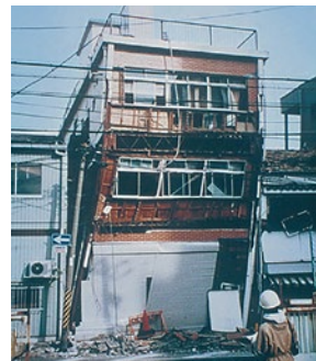
Abb. 2b: Kobe 1995. Foto: Architectural Institute of Japan
